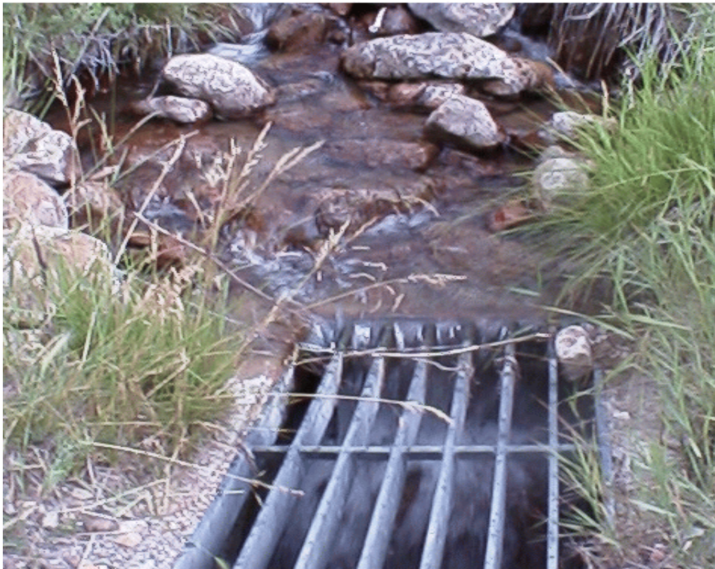
Figure 17. Upstream end of the US Highway 89 culvert on Twin Creek. Picture taken during low flows.
